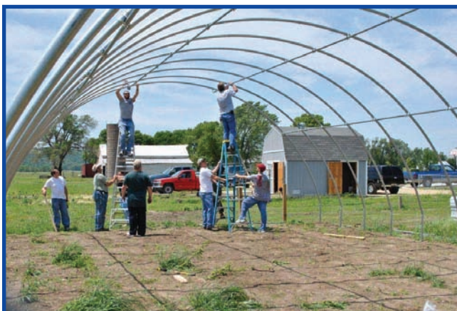
Construction of a greenhouse which will provide horticultural work opportunities for some of our clients was completed in the fall.
